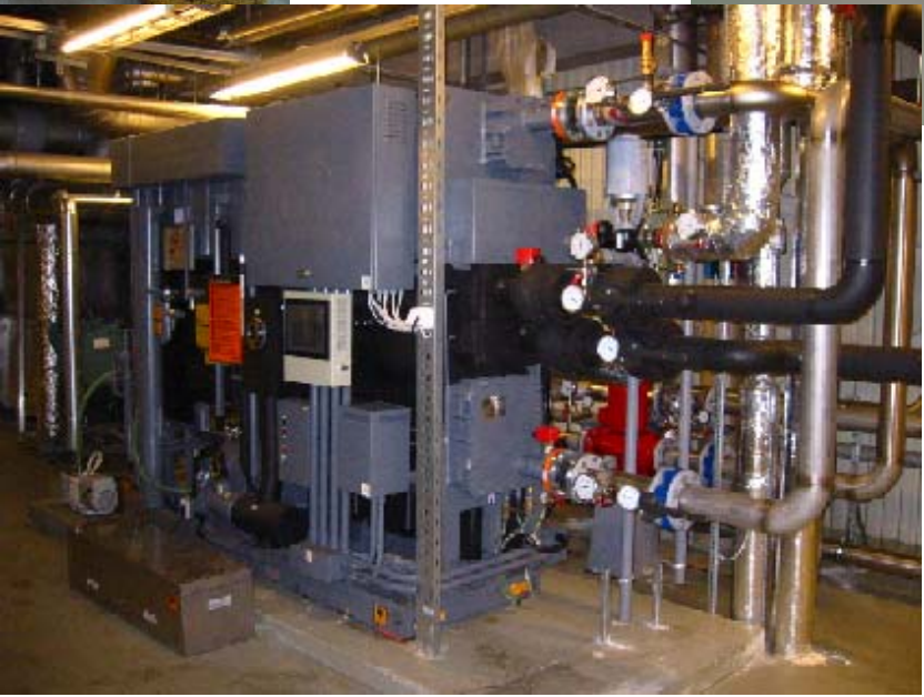
Broad Chiller at Statoil, Forus, Stavanger. Photo: Roar Stokholm, Statoil
