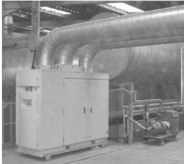
Courtesy: Bowman Power Systems [47]
