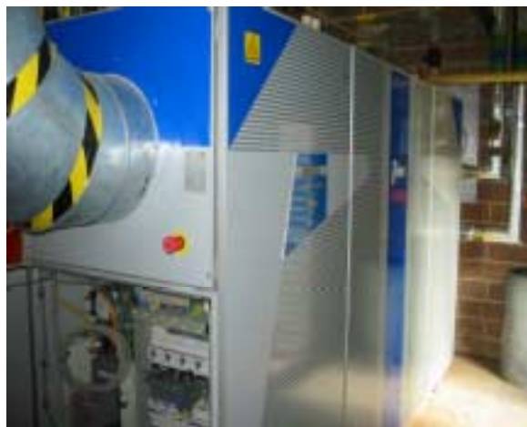
Fig. 20 The Turbec T100 gas turbine unit in-situ in the Kilmington WwTW engine house
