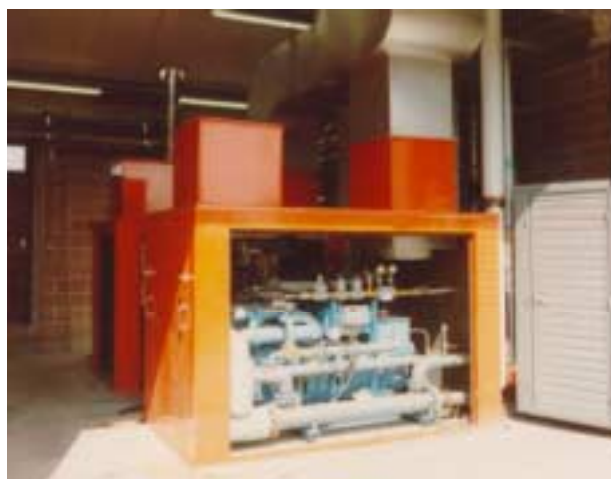
Fig. 19 The 30kW E reciprocating engines at Kilminster WwTW in-situ prior to removal
