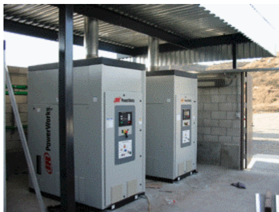
Figure 22, Ingersoll Rand microturbines at Jamacha landfill, California
