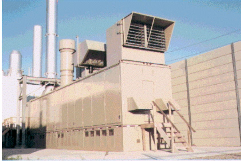
FIGURE 2: Steam Powered District Heating Cogeneration Plant
