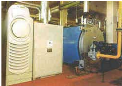
FIGURE 8: Capstone Microturbine - Generator System
