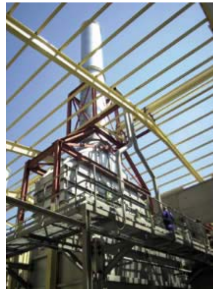
Cogeneration in Europe - part of a new, 10.6 MW cogen plant from Turbomach serving a food production company in Spain
