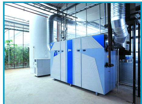
Fig. 7: Greenhouses CHP- Turbec T100 (by courtesy of Turbec)
