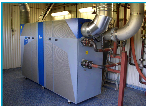
Fig. 4: Residential CHP-Turbec T100 (by courtesy of Turbec)
