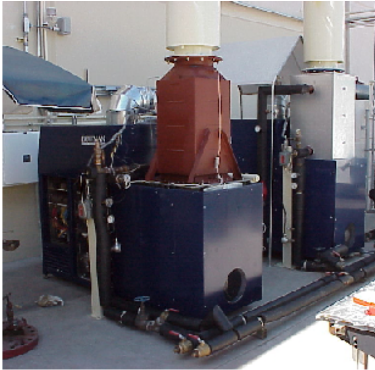
Figure 3. Bowman 60 kW (left) and Bowman 35 kW (right) MTG Units
